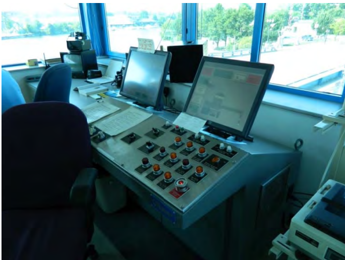
8 th Street Bridge Controls
