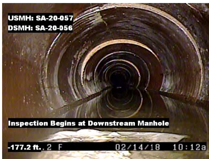
Debris in a Sanitary Sewer
