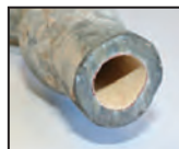
* The protective phosphate coating inside a lead lateral pipe.
