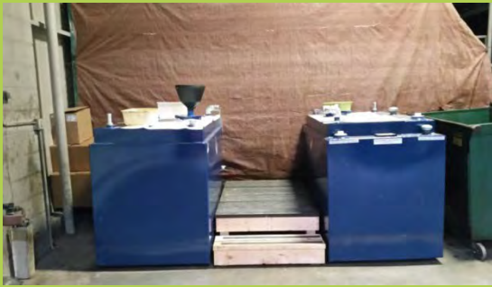
OIL COLLECTION TANKS
