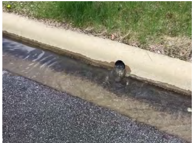
Incorrect Sump Pump Discharge
